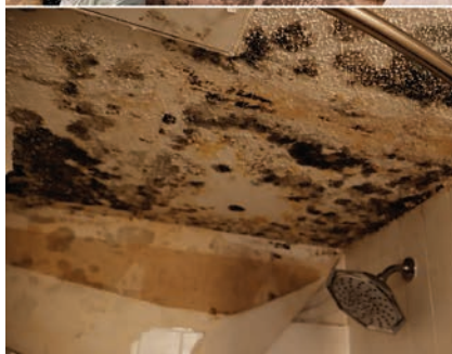
Devastating damage that went unrepaired by Mueller Flats landlords after Winter Storm Uri
